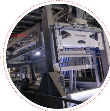
An automatic sack inserting machine (manipulator) in Huaxin Cement
