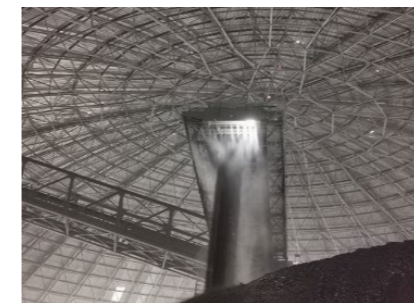
Yard Spray System
